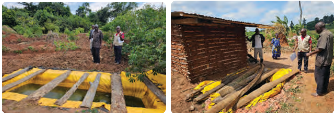
Figure 64: During the rainy season, an SAA RA farmer in Mubende, Uganda, harvests rooftop water from an improvised shed and stores it in low-cost underground reservoirs. The same farmer has constructed six such reservoirs around his farm to collect rainfall runoff, which he uses for irrigation during the dry season.
